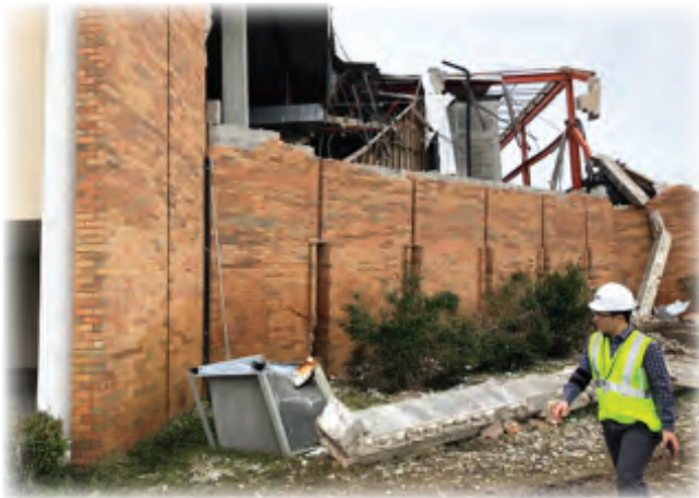
NIST staff in the field after Hurricane Michael. Photograph credit: National Institute of Standards and Technology.
